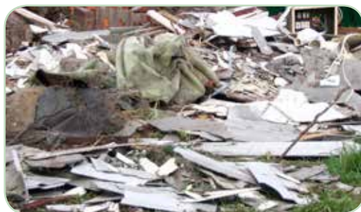
Broken asbestos cement materials from a demolition
