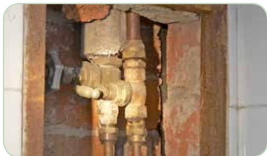
Friable asbestos lagging on pipes
