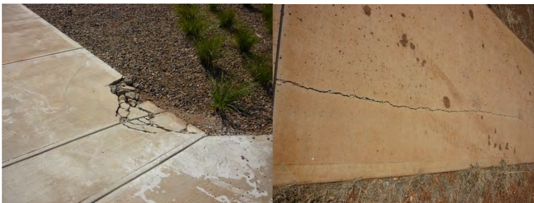
Figure 8 Examples of footpath deterioration adjacent to the site
