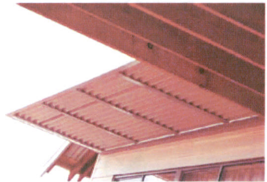
Example of good shading with overhangs and eaves (image courtesy of Rural Building Co) See 7.1.6, 7.1.7
